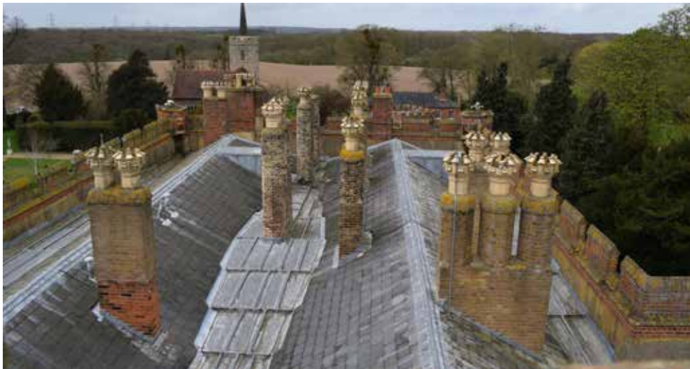
A1.4 – The view south incorporates the view of the Church that captures the important historical, religious and visual relationship between the two buildings and beyond, as in the other images is open countryside.
