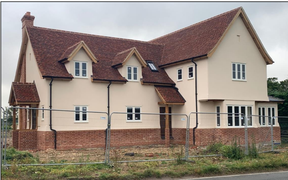
Figure 17: Homes under construction at Well Court in Hunsdonbury reflect roof lines and dormer features
